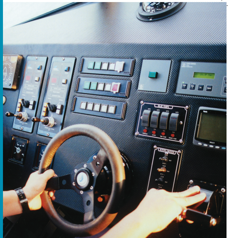
Typical MECS helm station.
